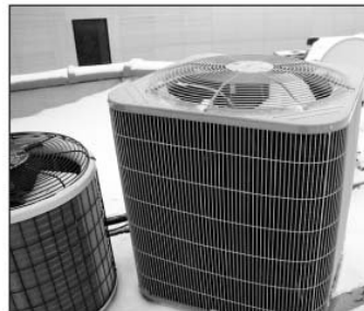
Air conditioning systems
